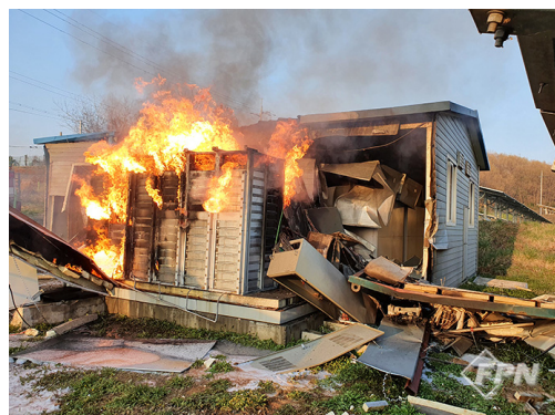
(a) Early-stage BESS fire incidents
