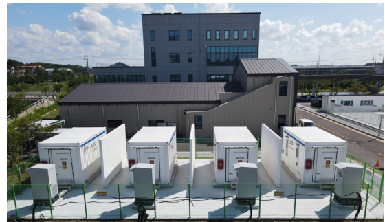
(b) On-site view of the demonstration facility
